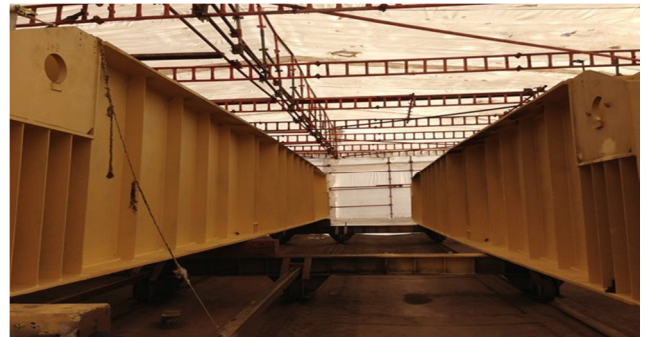
Figure 3 - Corrosion protection in dehumidified enclosures
