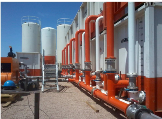
Figure 1 - Tanks installed in position, piping connected
