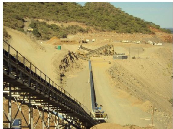
Figure 3: Overland coming from crushing plant
